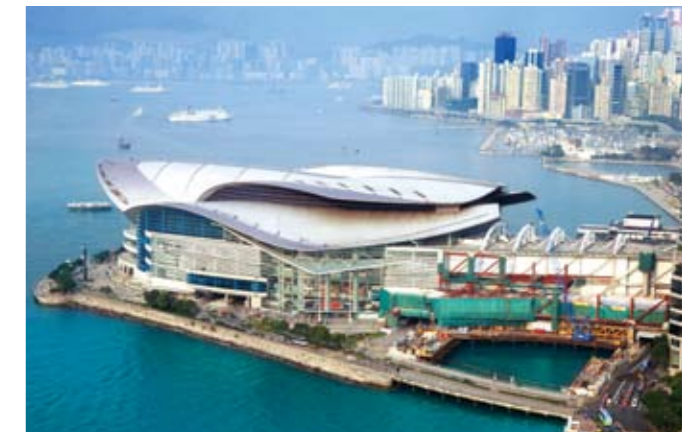
The HK$1.4 billion expansion to the HKCEC got going in May 2006. The three photographs (below) capture the expansion site in July 2006 (far left), late January 2007 (middle) and late March 2007 respectively.
